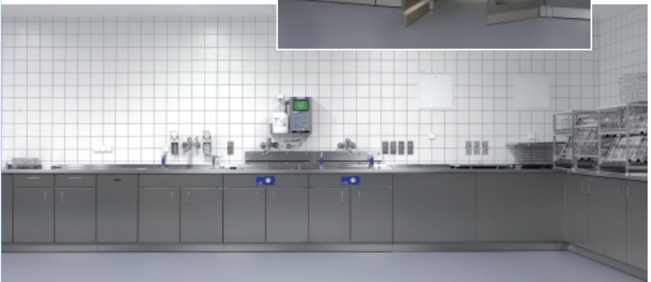
Central sterilisation unit Sterile material preparation unit made of stainless steel
